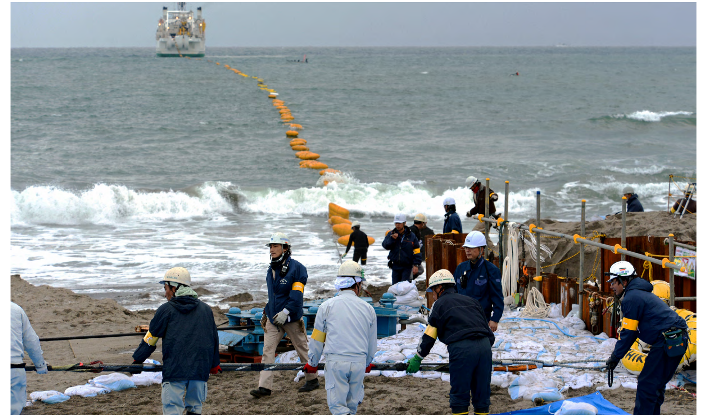
Workers pull an undersea fiber-optic cable from a ship, as KDDI Corp. began an operation to lay a cable connecting Japan and Singapore. Photo by The Asahi Shimbun via Getty Images
